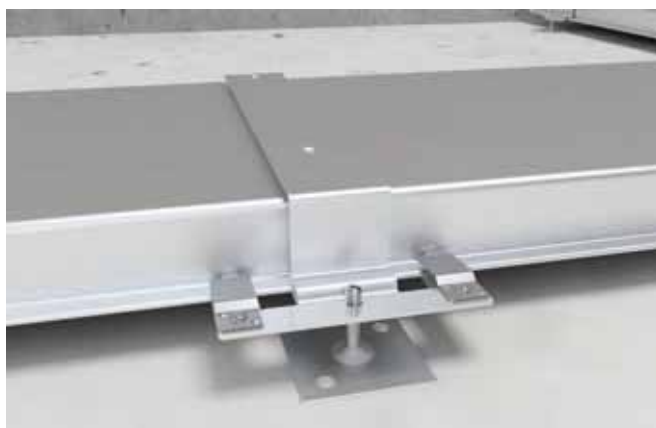
The usage of duct earthing element.
